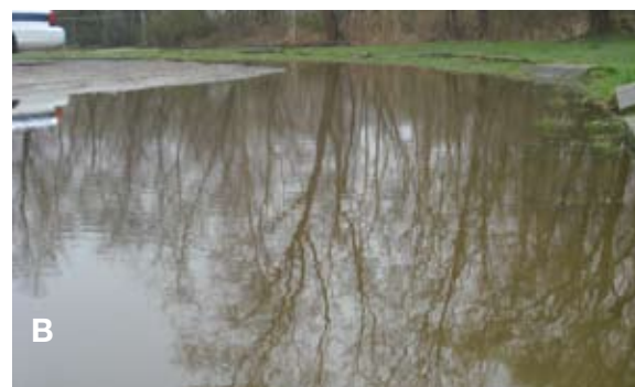
B: Puddling due to poor grading and maintenance.
